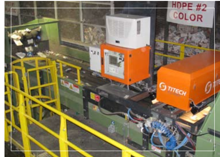
Rumpke Recycling, Material Recovery Facility (MRF) plastic sorting
