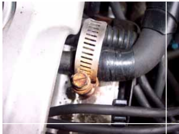
Example of an emission control system that has been tampered with.
